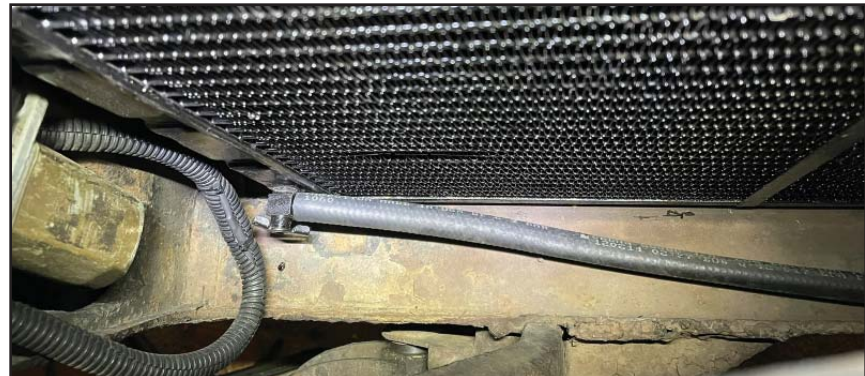
Looking down at the back side of the radiator, the orientation of the petcock and hose is apparent. The hose is long enough to reach into a drain bucket
