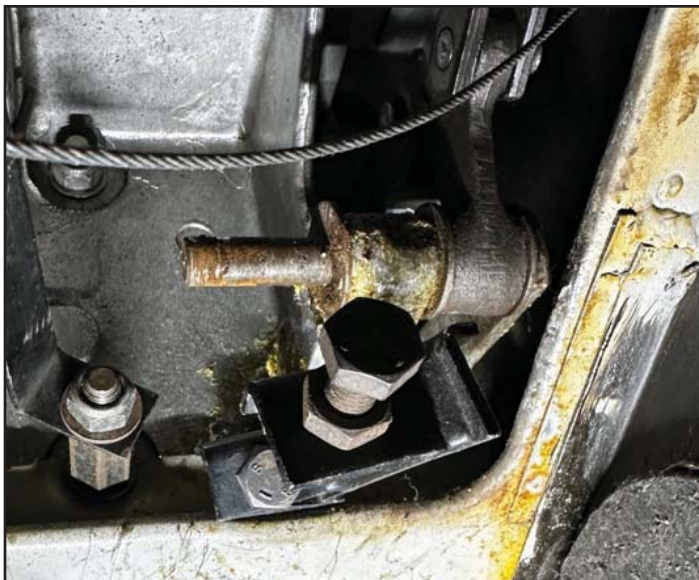
The shaft was covered with 50 years of dried grease and corrosion, which required extensive cleaning followed by lubrication
