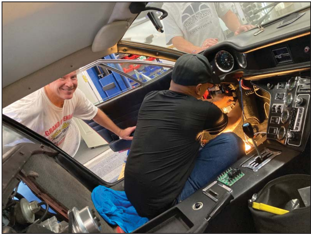
Sunday morning, and Paul is clearly happy, as Bayani Panis sets to work on the electrical system, installing more Pantera Electronics components
