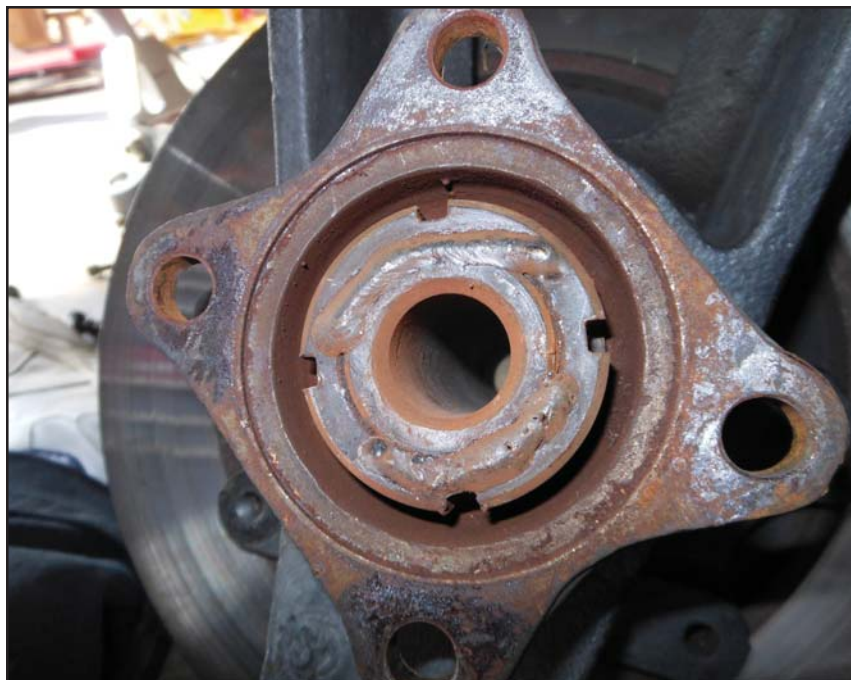
This is just plain evil. Some fool decided that the best way to secure the axle nut was to weld it to the axle!!!
